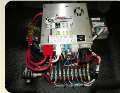
Wiring of WHELEN Cencom Siren Controller
